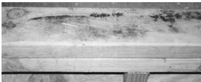
Fig. 1: Mold on lumber
